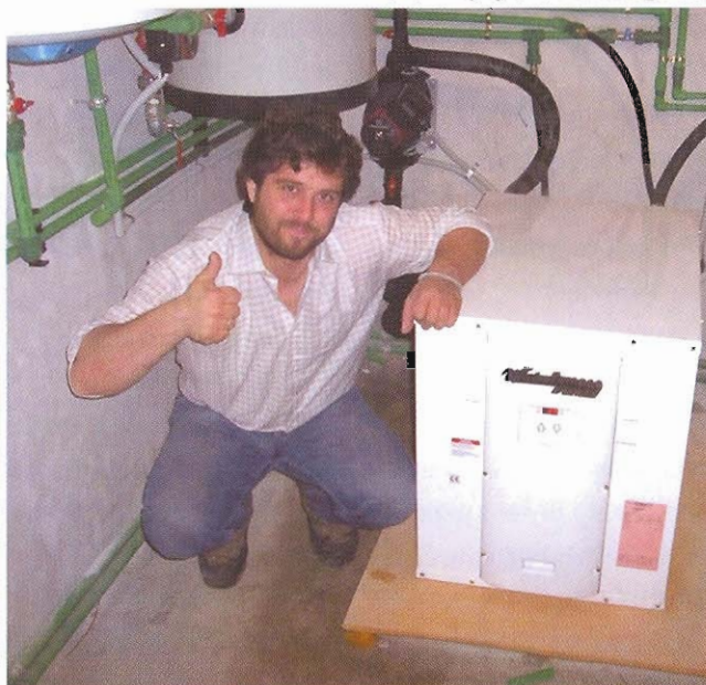
Homeowner, Sotirios Fanis, signals that all is well as his ground source heat pump system and WaterFurnace unit starts up for the first time.
